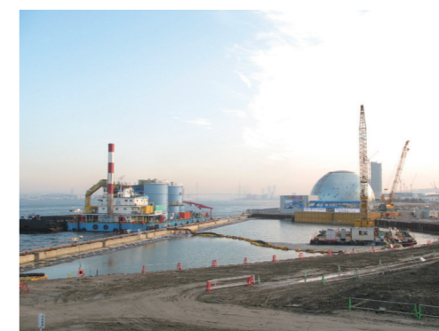
Reconstruction work of the embankment of Yumesima Immersed Tunnel at Osaka Port
