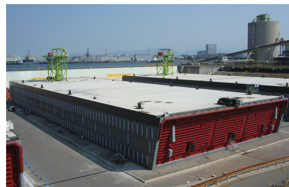
The 11th National Land Technology Development Award Grand Prize, Key Element Construction Method (New method for connecting immersed tunnel elements without the works of the last coupler as is needed in a conventional method)
