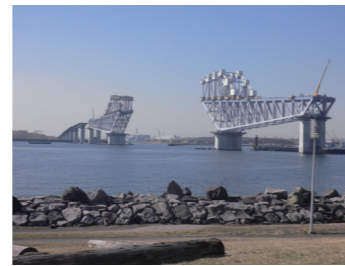
Tokyo Gate Bridge (under construction) (Photo: Tokyo Port office, Kanto Regional Development Bureau, Ministry of Land, Infrastructure, Transport and Tourism)
